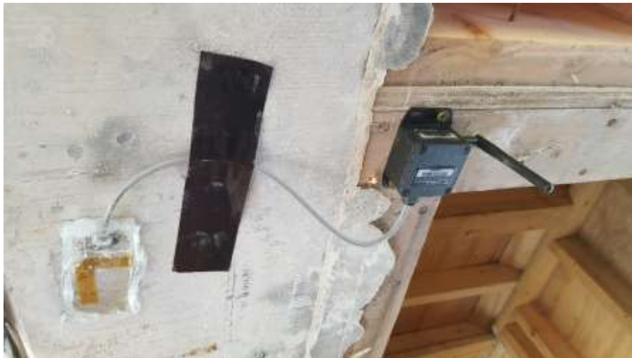
Figure 7-5 Installed SenSpot Strain Gauge
