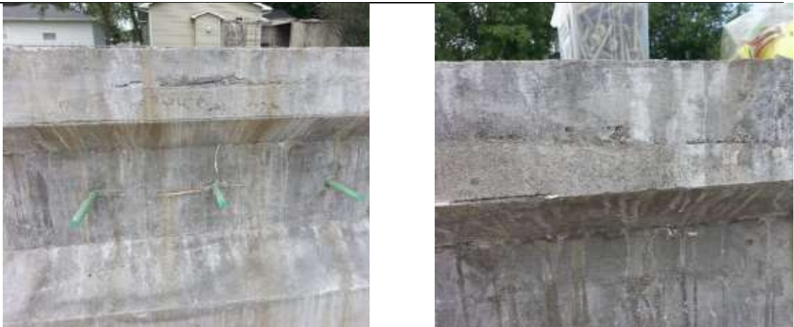
Figure 5-13 Cold Joints Appeared on Second Girder
