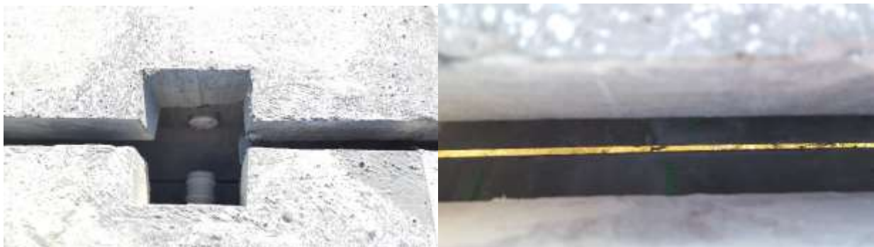
Figure 5-30 Gaps Created at Each Joint
