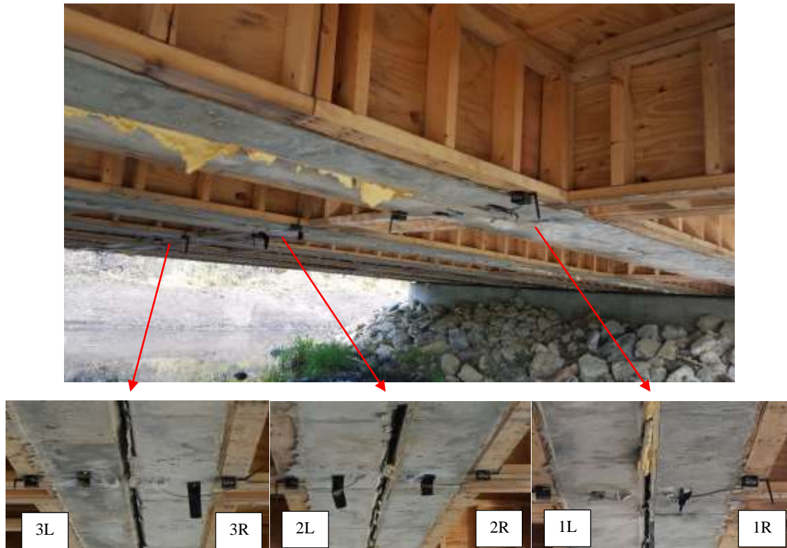
Figure 7-6 Installed SenSpot Strain Gauges
